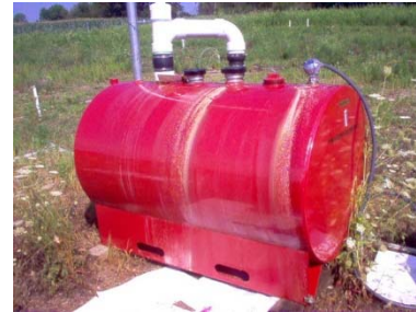
One of the overfilled ASTs
