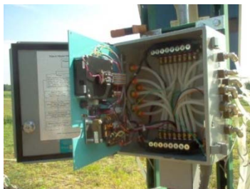
Inside of the pump control panel
